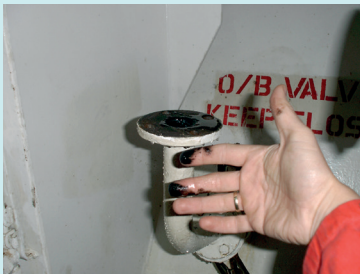
Oil found in overboard valve
