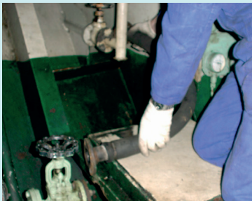
Illegal pipe – sludge pump to overboard
